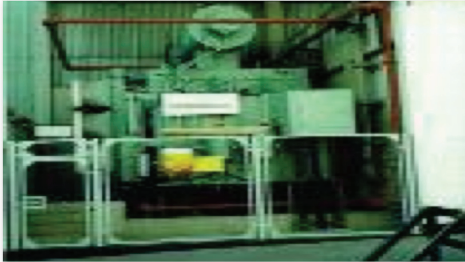
Fig.33: Example of oil-filled transformers room
