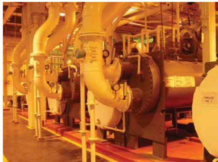
Central Chiller Plants
