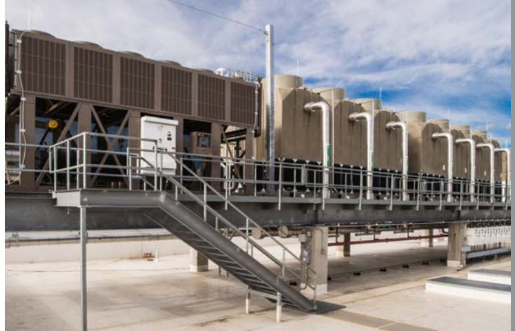
Johnson Controls thermosyphon with hail guards and cooling towers on top of the ESIF. Photo by Dennis Schroeder, NREL 41999
