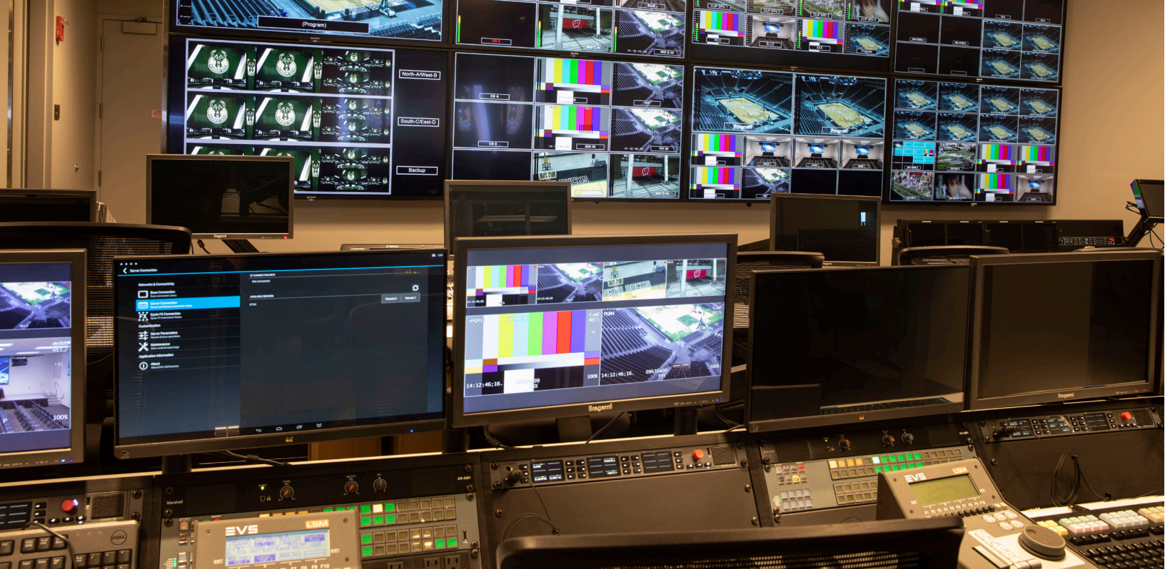
Video Control Room
